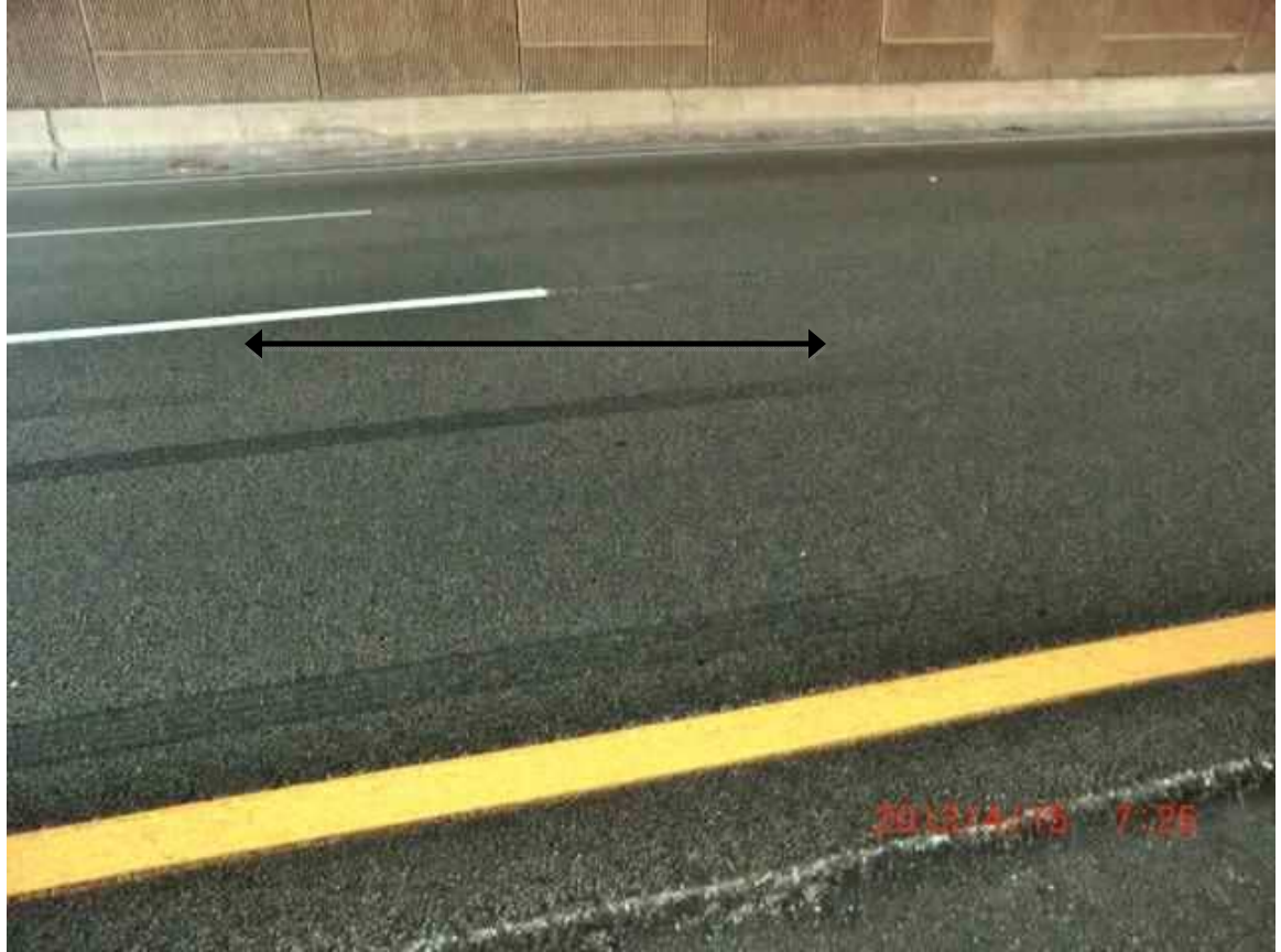
Beginning of skid. Note the distance between the first and second set of skids measured at 8 ft.
